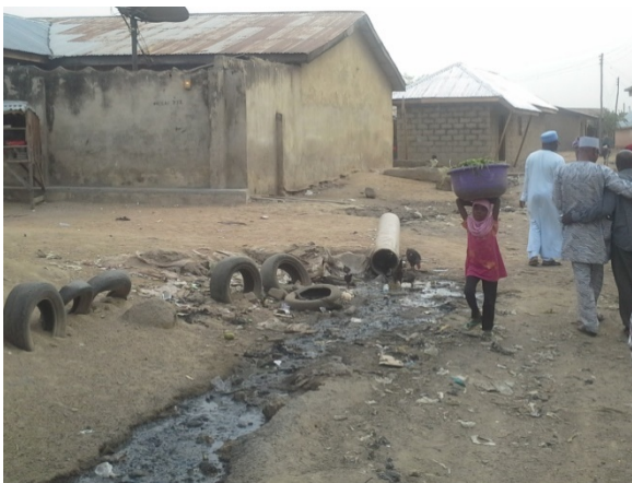
Fig. 2: Unplanned drainage cutting through the road Barkin-Sale area of Niger State, Nigeria (Source: Author's fieldwork, 2013)
