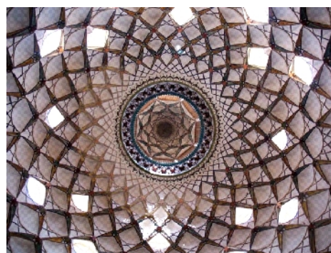
Fig. 18: Openings in the middle of Yazdi-bandi units across the ceiling, Boroujerdi-ha house
